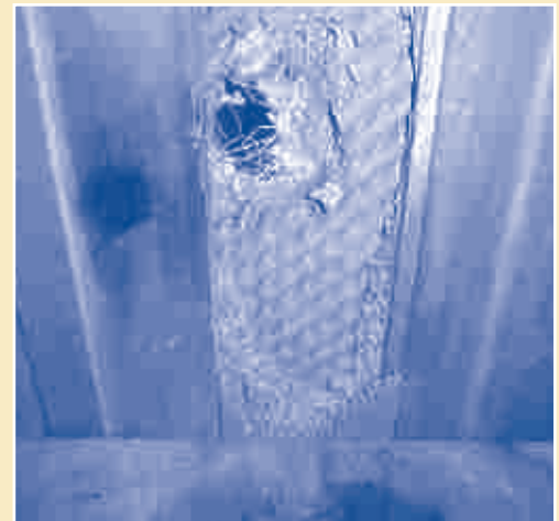
Hole in floor as viewed from basement Survey 2004
