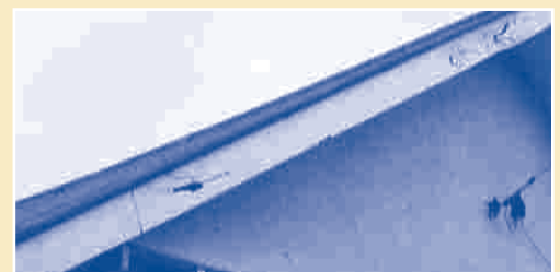
Rotten surfaces allowing water to leak in, Survey 2004
