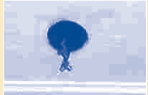
Ceiling hole, bare wires and no lights Survey 2004
